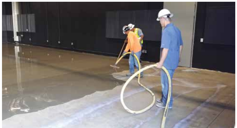
Figure 6. Installation of a cement underlayment in which the thinness of the application can be observed. Prior to installation, the concrete subfloor had to be shot blast to ensure adequate bonding of the underlayment.
