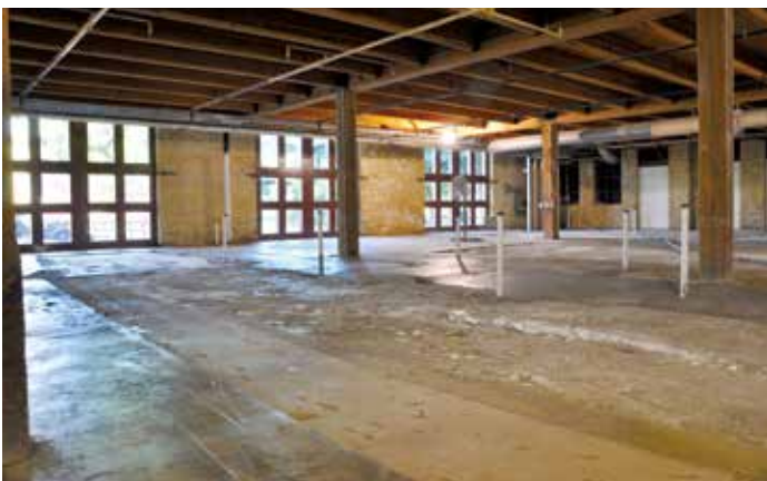
Figure 3. The floor of this train station needed significant work prior to repurposing. In this photo, extensive floor height variations can be seen in the locations where tracks were removed.
