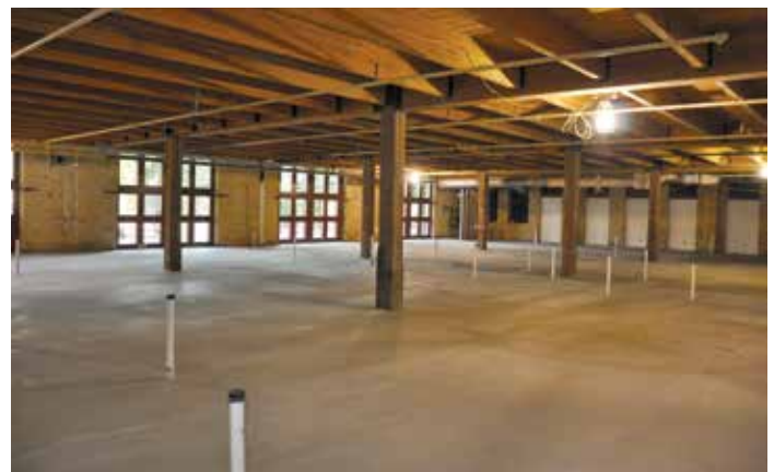
Figure 4. The same area is pictured following the installation of a high-end gypsum underlayment, which leveled the floors and created a smooth surface ready for floor coverings.
