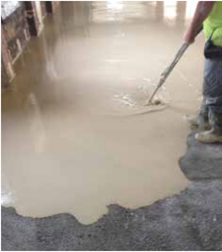
Figure 2. In this project, a lightweight deep-fill screed was installed and allowed to dry overnight. The next day, the hardened screed was topped with a gypsum underlayment to provide the density and compressive strength needed for point load dispersion and floor bonding compatibility.
